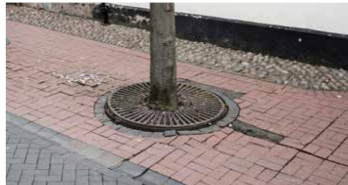
Paving effected by root heave (above)
